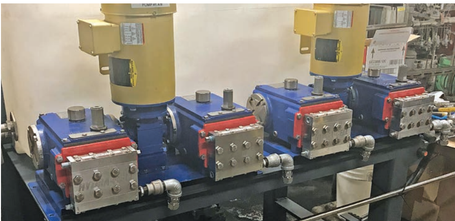
Chemical boiler feed at a power plant. Four MT8 pumps running off two gearboxes and two motors shows its duplexing capability.
