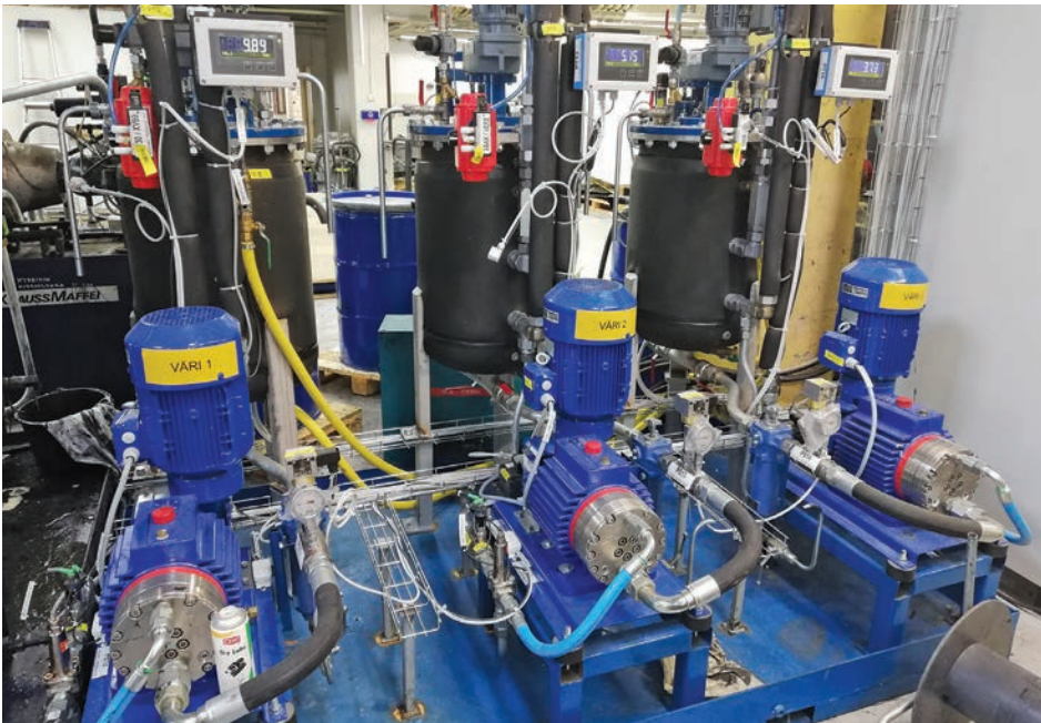
Three P500 models replaced six piston pumps for spraying an adhesive colorant and substantially reduced maintenance costs.
