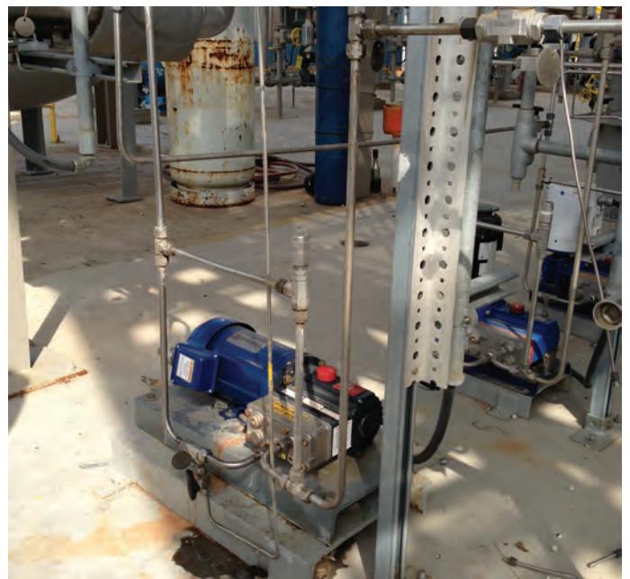
Hydra-Cell pumping ethanol-based fluid for making jet fuel.
