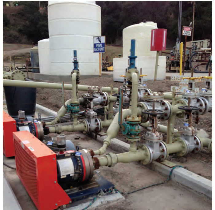
Several operational features of Hydra-Cell pumps are showcased when processing volatile crude oil.
